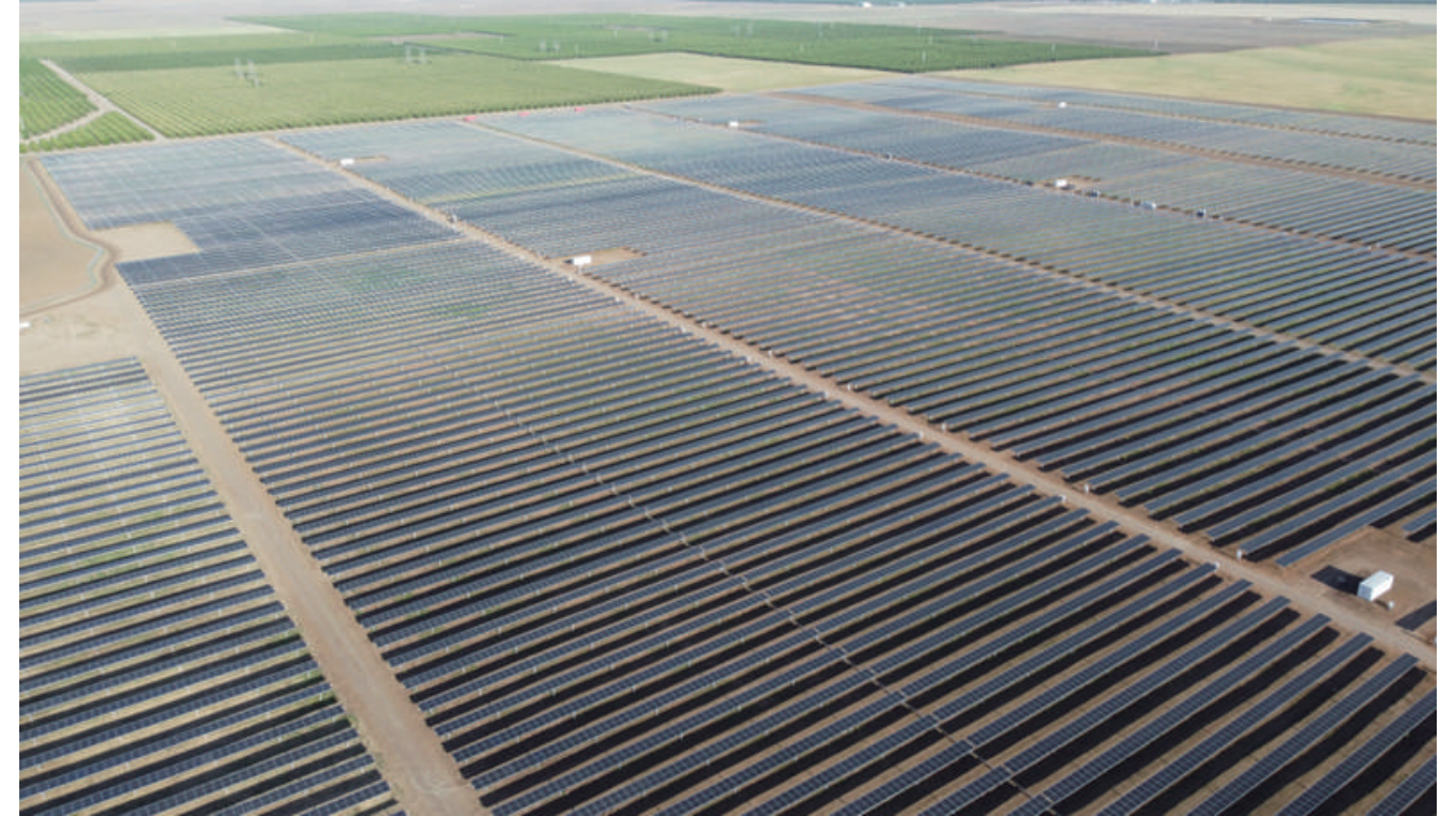
• 73MWp Tulare County,California,USA
